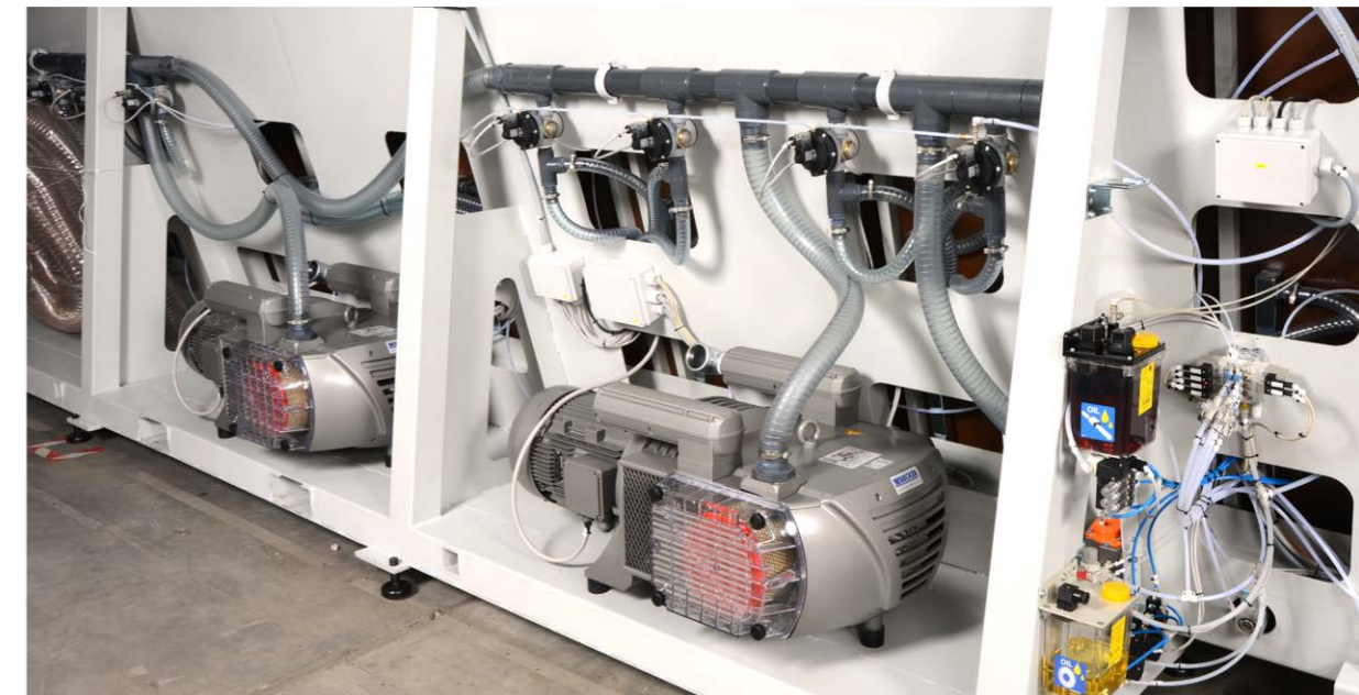
Dry vacuum pumps (Made in Germany)
